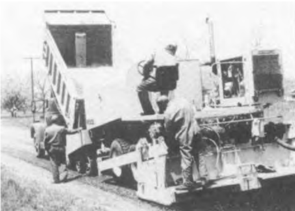
Figure 4-45. Hopper-type pugmill travel plant.
