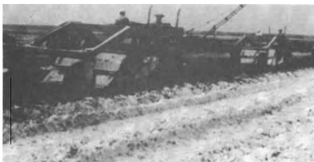
Figure 4-38. Train of rotary mixers.
